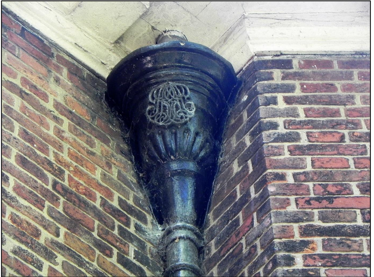
Fig 19 Decorated drainpipe head to the east of the bay window.
