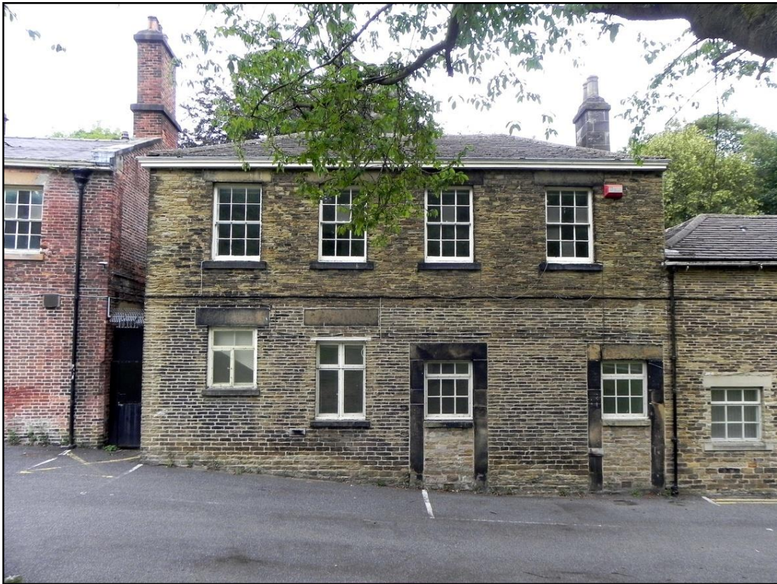
Fig 5 Detail of the south elevation showing the two doors, now blocked up and reused as windows.
