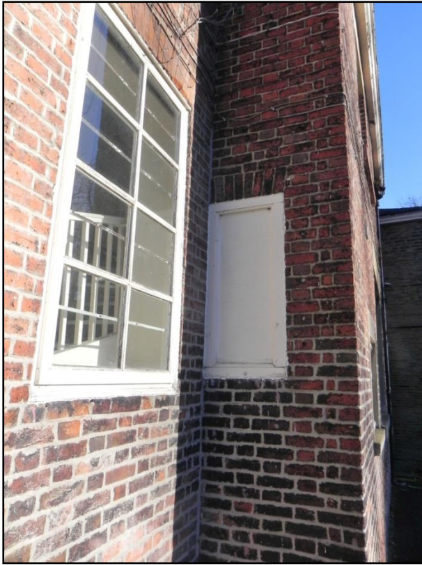
Fig 7 The blocked-up window in the west wall, which provides stratigraphy between the buildings.
