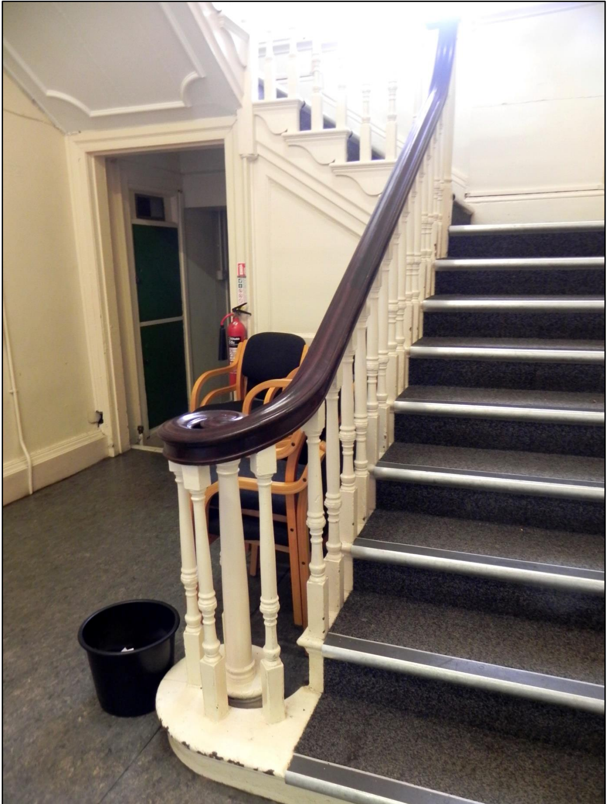
Fig 17 The bottom of the staircase showing the curtail step.
