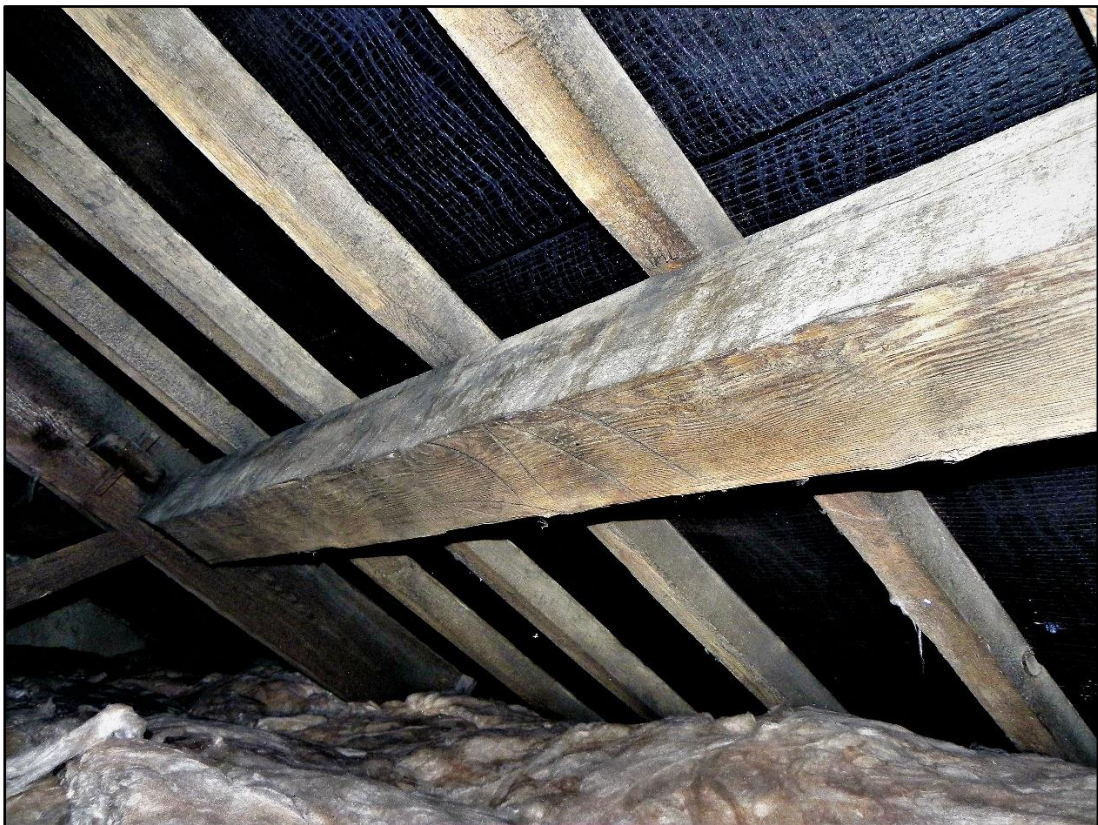
Fig 28 A marking found in the roof void which had not been painted.
